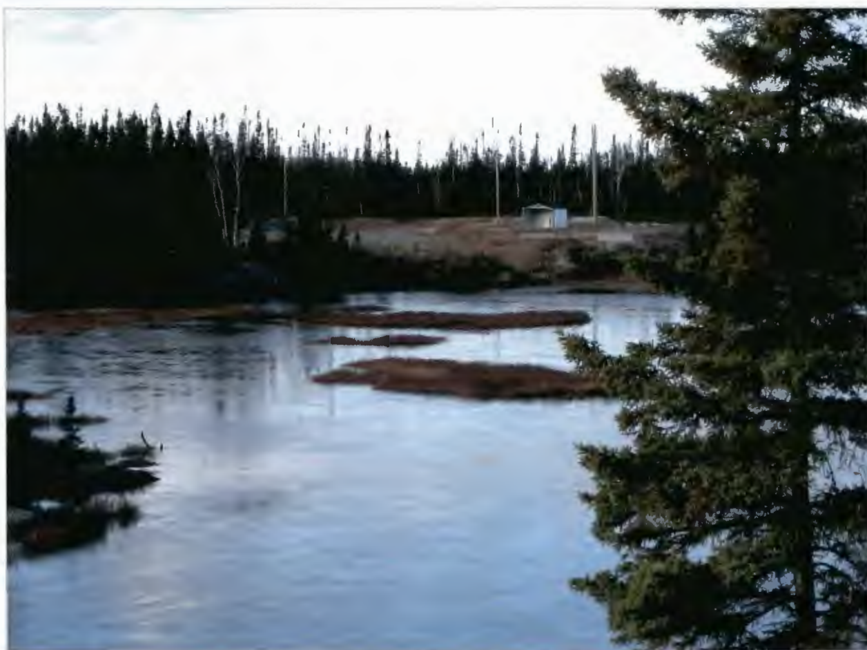
Figure 3. Capped winze and ventilation shaft above the Pick Deposit on Orebot's Claims.
