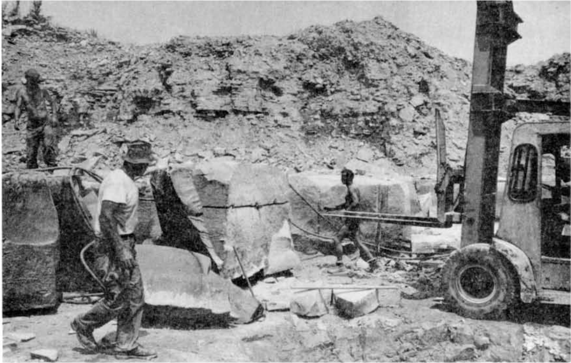
Fork lift truck used to lift blocks of sandstone at Structural Sandstone quarry, Glen Williams.
