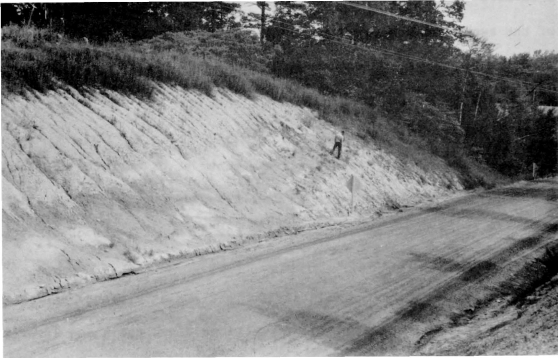
Photo 3. Road cut exposing Leaside Till over sand. Dufferin Street, north of Maple Road and near Department of Lands and Forests Research Station.
