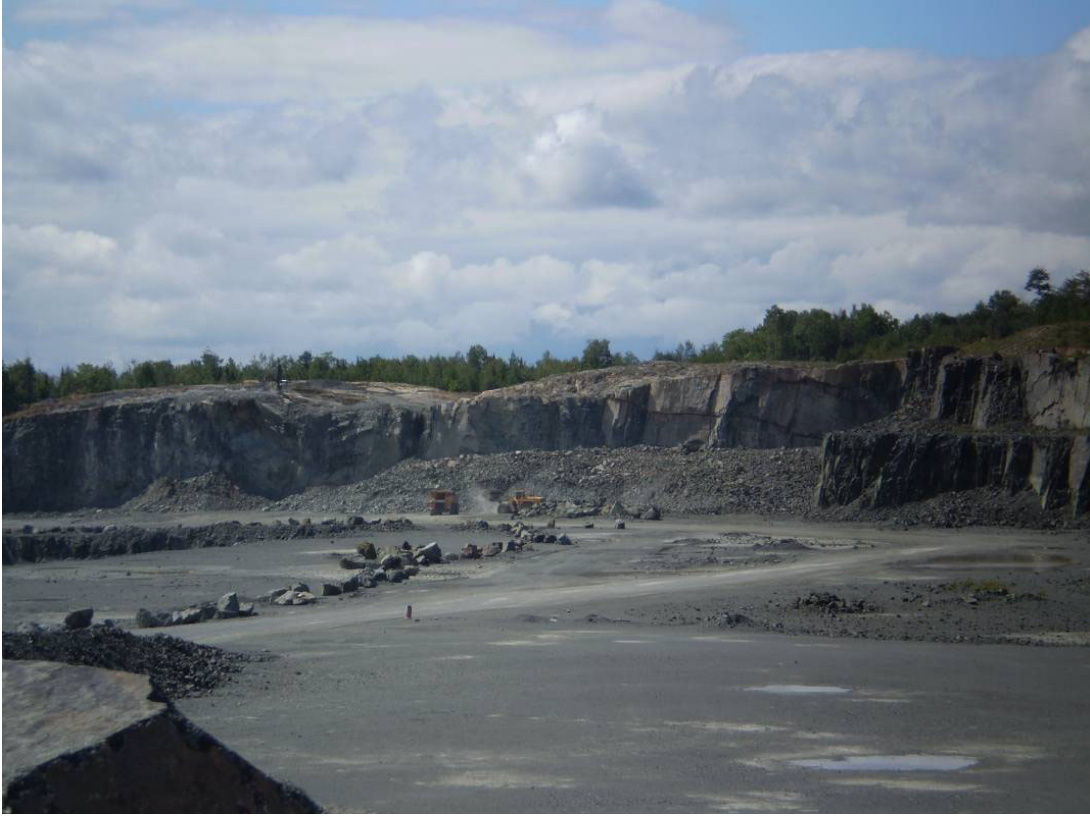
Figure 1. Extraction of trap rock from the Nipissing diabase located in Bruce Mines during a recent property visit by the staff of the Sault Ste. Marie Resident Geologist Office.
