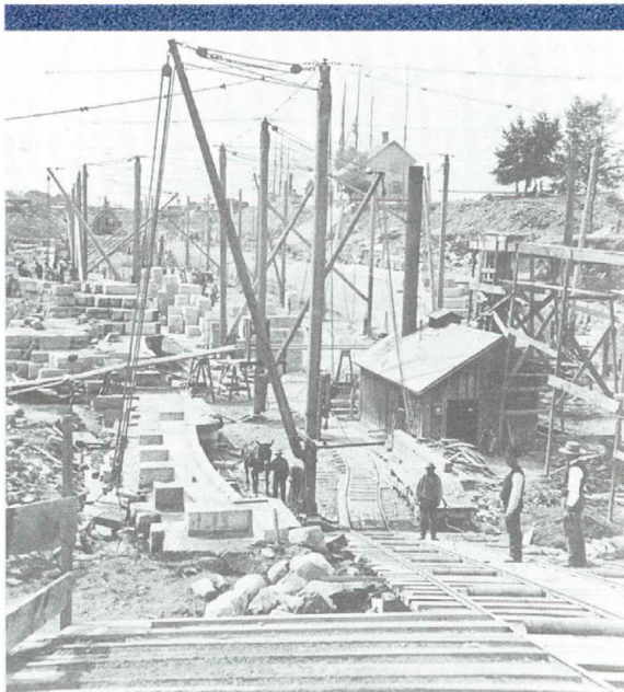
PHOTO 125: Construction on the Canadian locks at Sault Ste. Marie began after the US refused a Canadian ship passage through the American locks in 1870. The locks, shown here under construction ca. 1880, were completed in 1895.
